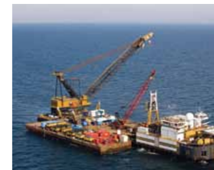
Atlas Copco industrial rental compressors in action during pipeline pre-commissioning in deep water.
