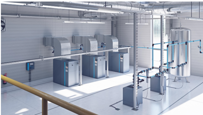
Installation with external dryers
