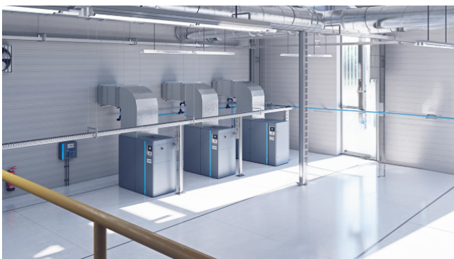
Full feature installation
