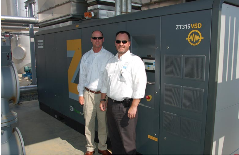
Left to Right: Carl Kline (Haas CNC Racing) and Jim Bruce (Atlas Copco) with the on-site oil-free rotary screw compressors at Windshear Inc.
